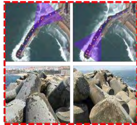
Fig. 1. Systematic photographs taken at predefined point 6 of Ericeira's breakwater, according to two predefined directions (northeast-left and southwest-right).
